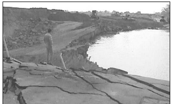
Figure 4. Sliding mass as seen from the wharf.
